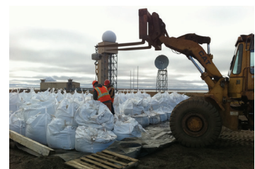
An Olgoonik subsidiary company performing government contract remediation work at the old DEW Line site.
